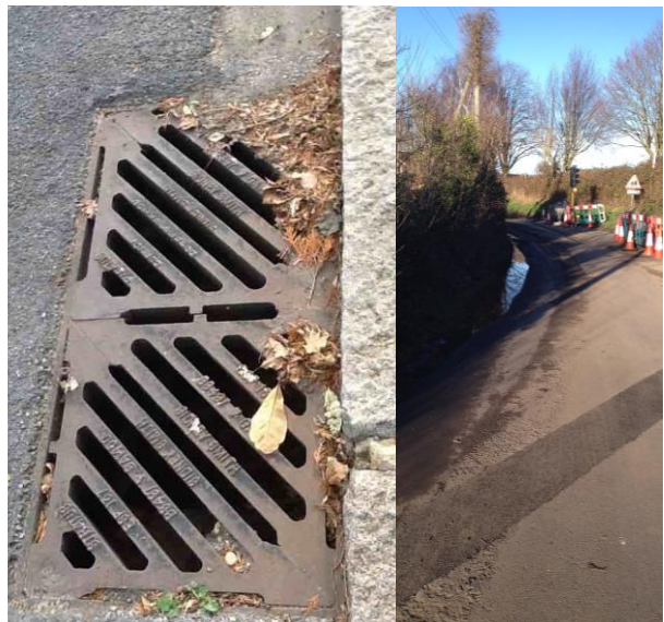
No action required: Intervention level not met
